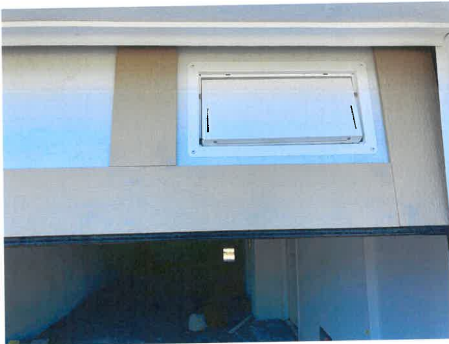
Photo One Caption Garage Door Vent 12/08/2020
